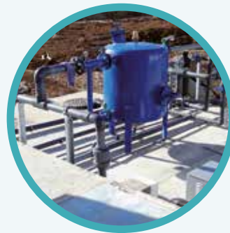
Filtration unit of the SBR.
