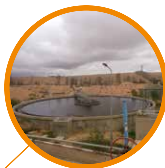
Existing treatment facilities of Médenine Wastewater Treatment Plant.
