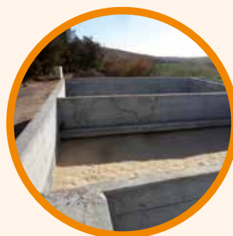
Constructed sand filter of Médenine Waste Water Treatment Plant.
